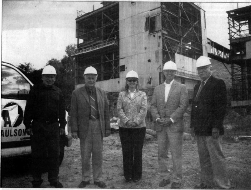
Aulson Company demolition experts are onsite at the former Franconia Papermill in Lincoln to begin dismantling the local landmark. On hand for the beginning of the end of the Mill Era in Lincoln is, from left: Dennis Ducharme, developer and president of RiverWalk at Loon Mountain, LLC; Executive Councilor Ray Burton; Tara Reardon, NH Department of Employment Security Commissioner; Kevin Clougherty, NH Department of Revenue Administration Commissioner; Roger Sevigny, NH Insurance Commissioner. After decades of disuse, the papermill is being removed to make way for the development of a new 170-unit resort hotel, bringing an estimated 100 jobs to the area.
